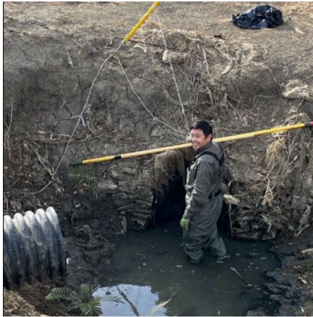
Solano RCDs, Kevin Young-Lai, assistance with the removal of an animal trap lodged in a culvert.
